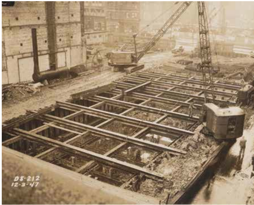
Measurements from instrumented excavations during subway construction in Chicago formed the basis for Wu's PhD thesis "An Analytical Study of Earth Pressure Measurements on Open Cuts," under the supervision of Ralph Peck.
